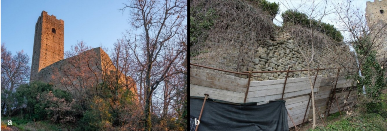
Fig. 1. The fortress of Larciano a), and part of the eastern wall before the restoration b). Vegetation, collapses, safety precautions and the steepness of the ground are visible (© Chiara Marcotulli).
